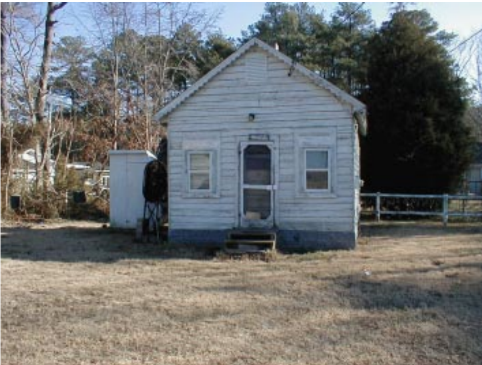
Home, located in Metompkin, without indoor plumbing included in the project grant.
