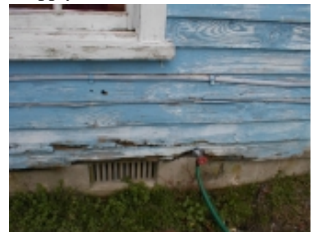
Lead Paint Hazard
