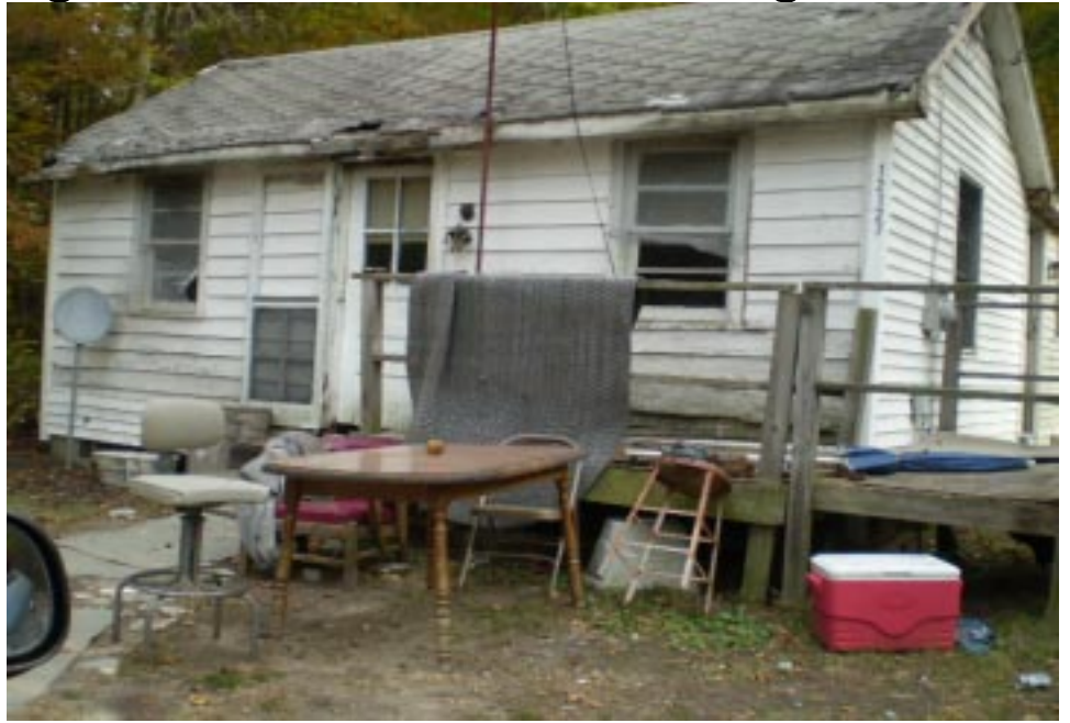
House lacking indoor plumbing
